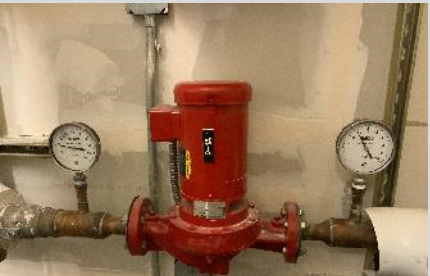
Chilled Water Pumps
